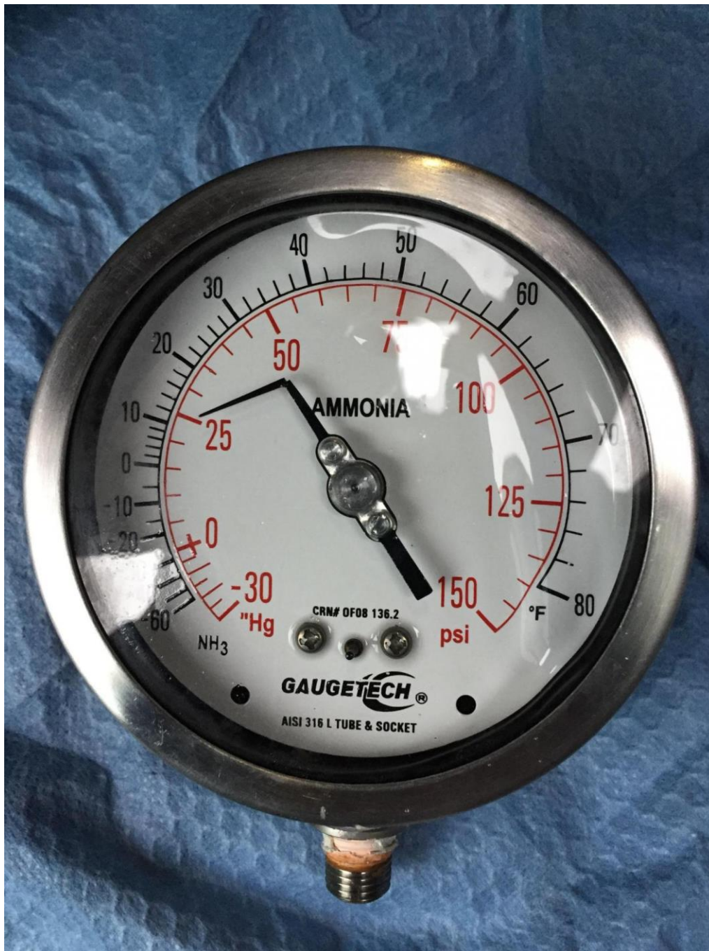
Photo 3: Broken ammonia pressure gauge – needle is broken at location of stopper pin and internal calibration mechanism shows deformation or offset.
