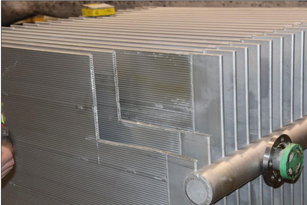
Figure 7 Bulged plate removed from 2 nd row.
