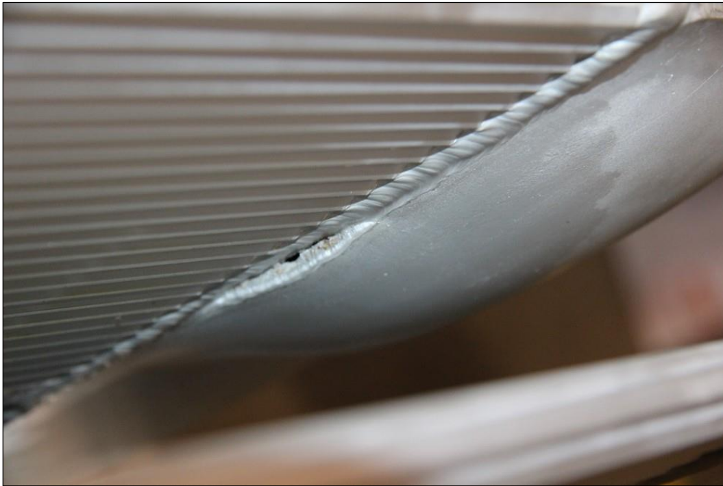
Figure 5 Weld tearing at bottom of bulge opposite (see Figure 4).
