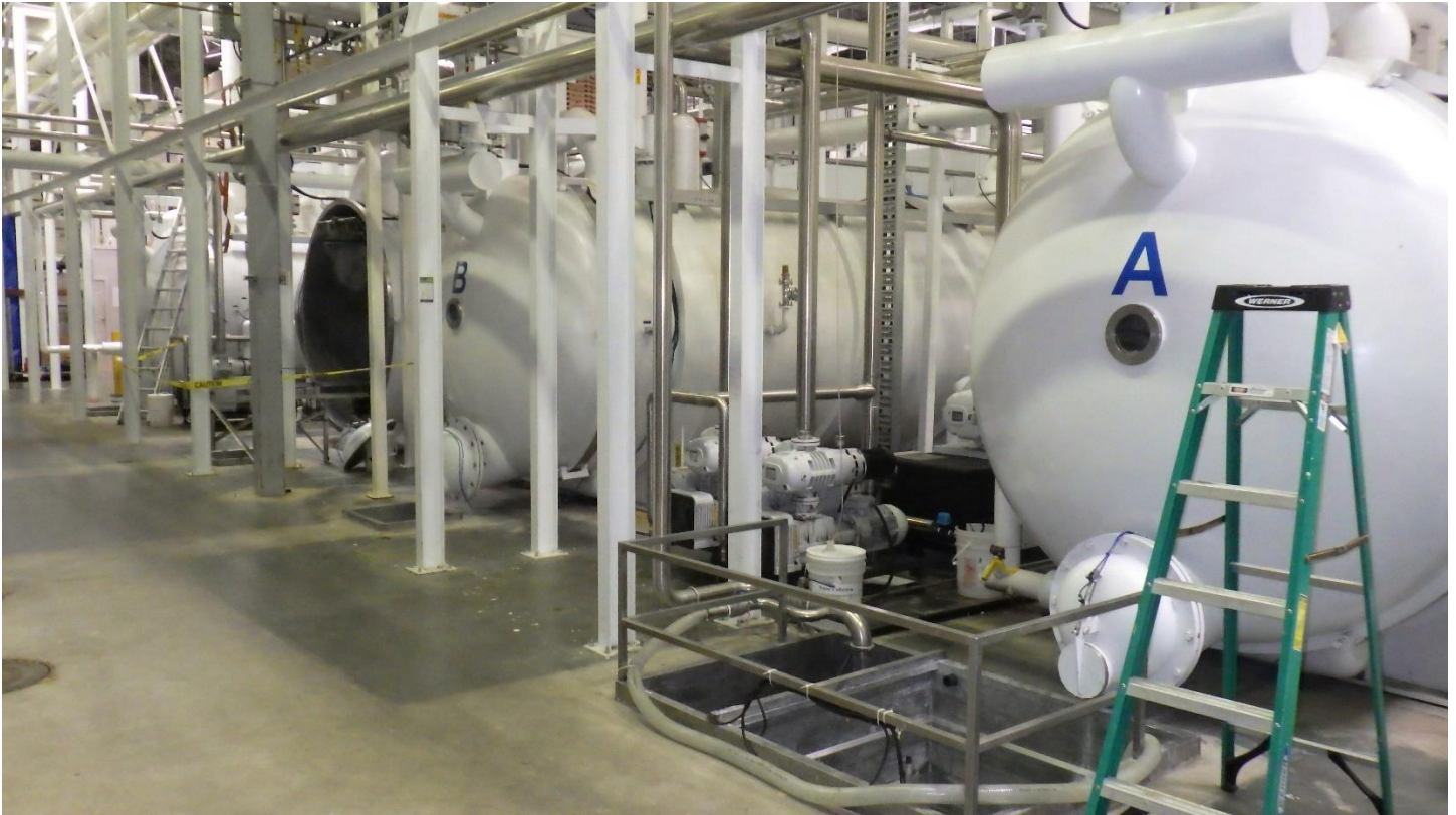
Photo 4: Freeze drying chambers at processing facility. Labels visible on chambers A and B while access door is opened on chamber C.
