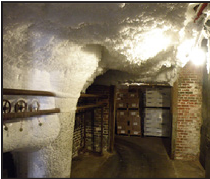
EPA inspection photo reveals dangerous ice buildup on ammonia piping and valves.
